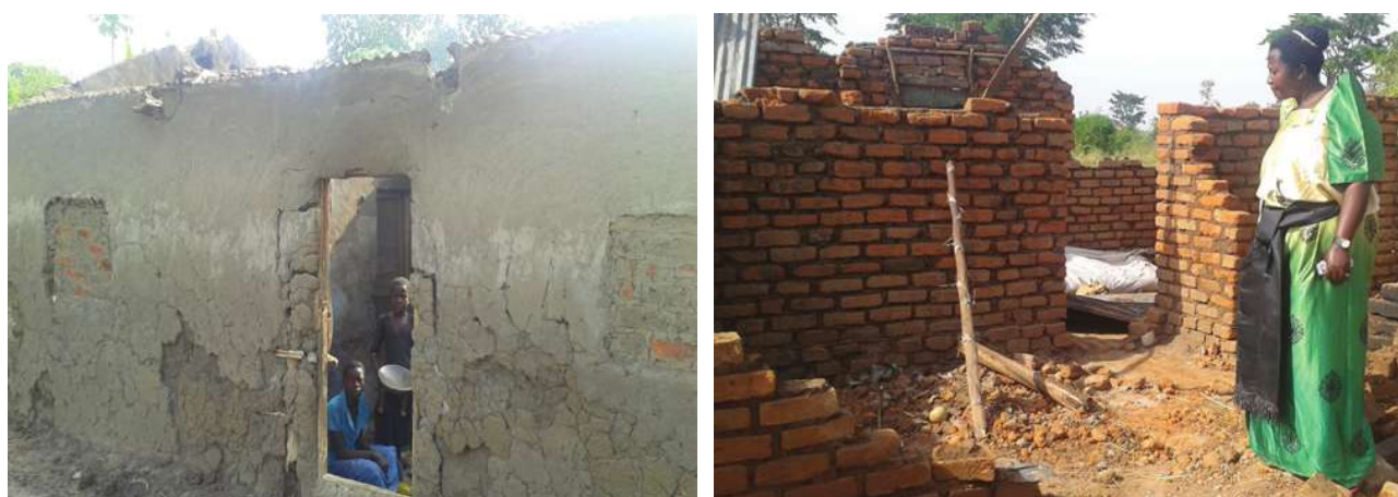
Plate 5: Houses destroyed by strong wind and hail storms in Himutu
